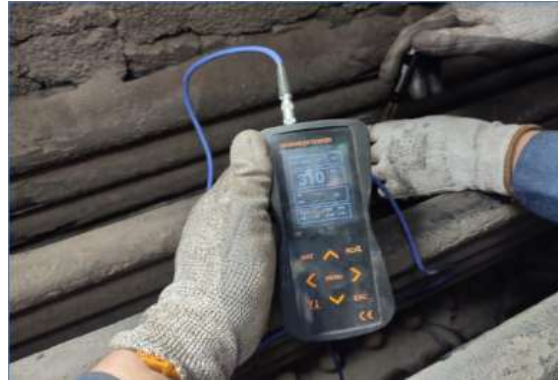
Figure 10 Hardness testing on Water Tube compartment 1
