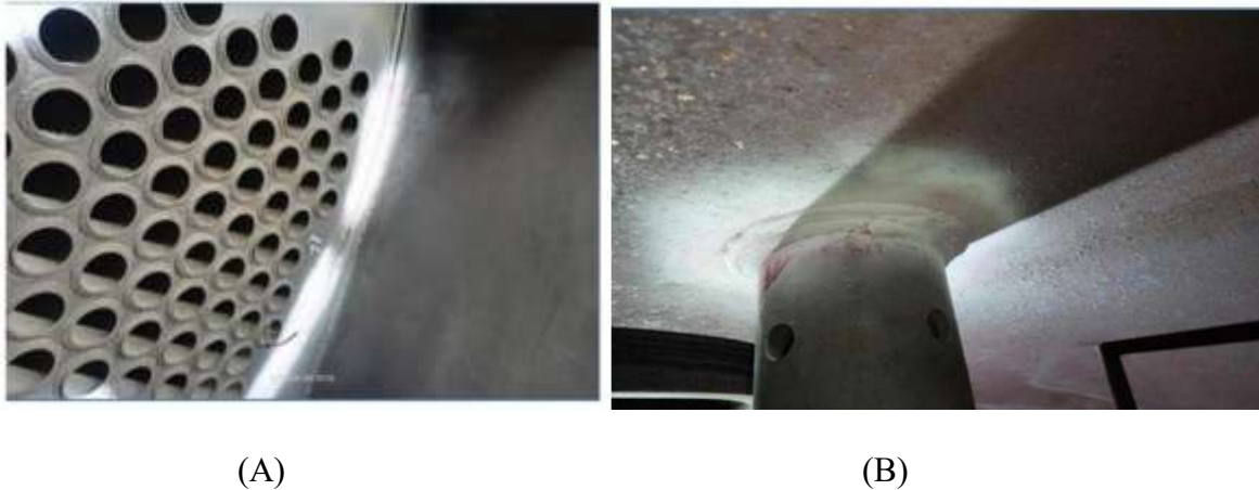
Figure 8 (A). Dye Penetration Test on Tube Sheet (East) and (B) Dye Penetration Test on Nozzle
