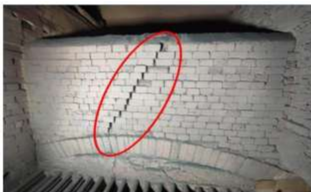
Figure 6 Cracks in the wall in the furnace area in the partition area.
